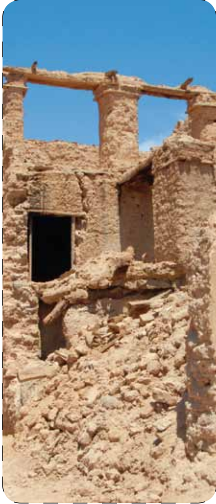
Observation of construction systems and pathologies
